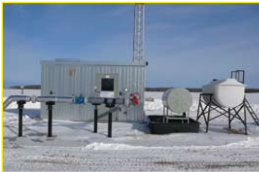
Typical Elmworth Wellsite Facility
