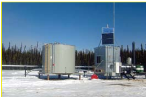
Saxon Wellsite Facility with Lineheater and Telemetry
