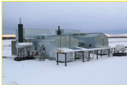
Elmworth Compressor Station – Second compressor installation alongside original compressor.
